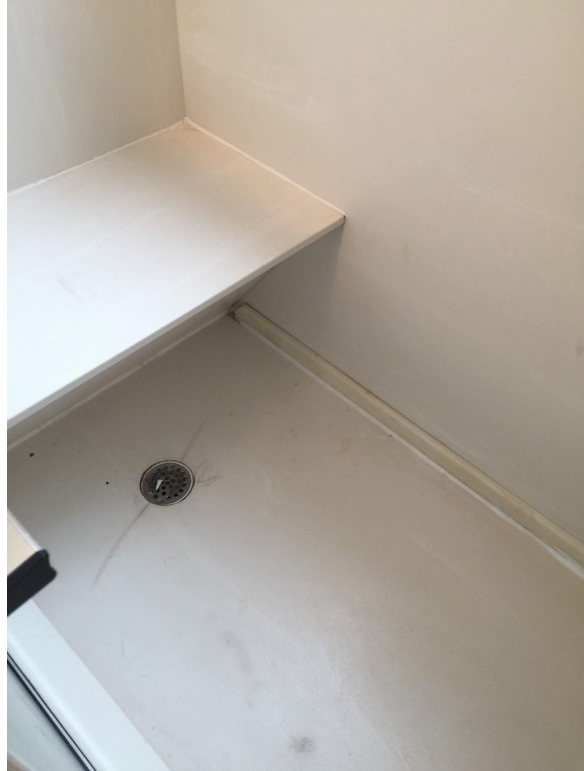
Close-up example of an older cultured marble style and surface wear.
